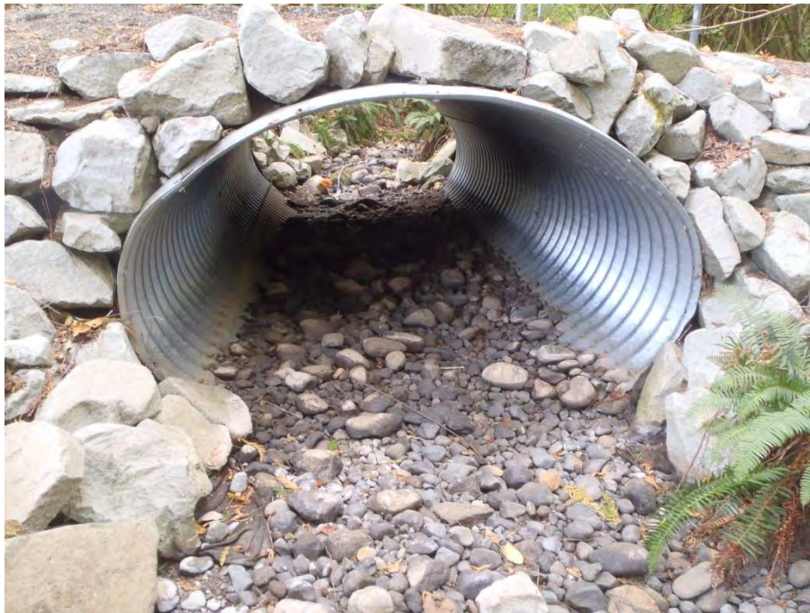
Photo 5. View upstream of the existing pedestrian trail culvert crossing across Piercy Creek mainstem located near the southern property boundary. (Aug. 30, 2017).
