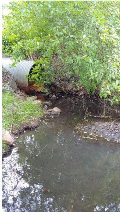
Label Photo 6. Culvert running south beneath subject property, through which Stream 2 flows southwest. Photo taken from Stream 1, which flows northeast toward culvert.
