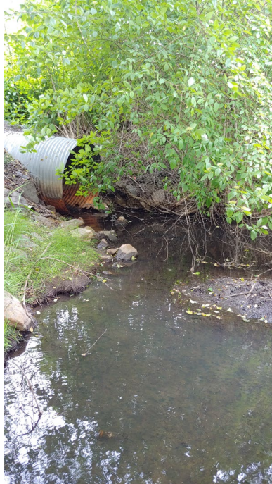
Photo 8. Culvert running south beneath subject property, through which Stream 2 flows southwest. Photo taken from Stream 1, which flows northeast toward culvert (June 2020).
