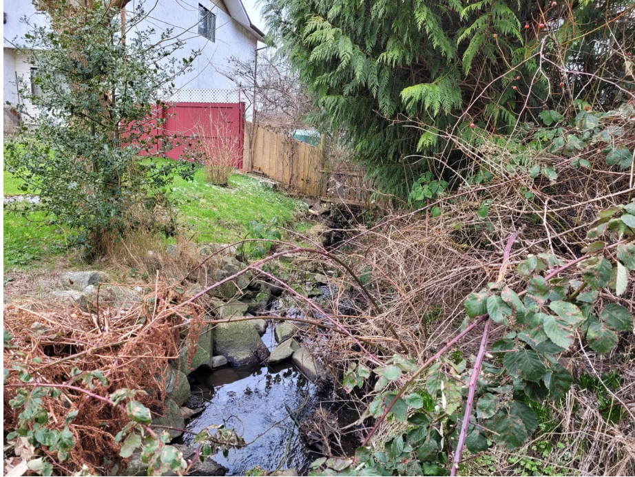
Photo 19. Bonner Creek downstream of 2.2 m diameter culvert. Creek flows beside residential properties and has armoured banks (February 2021).
