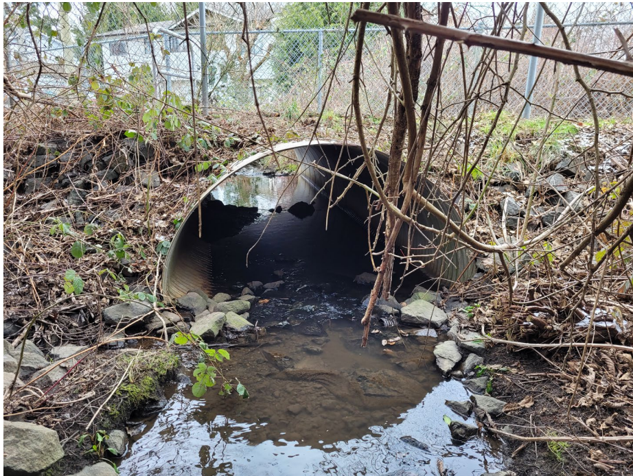
Photo 18. Bonner Creek flows through a 2.2 diameter CSP culvert beneath walking path to Williams Road, looking downstream (February 2021).
